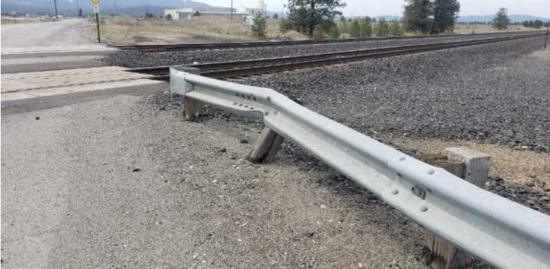
IMAGE 33: Idaho Rd southbound guardrail damage at rail crossing
