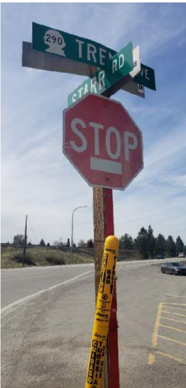
IMAGE 27: Starr Rd southbound, faded stop sign, bent signs
