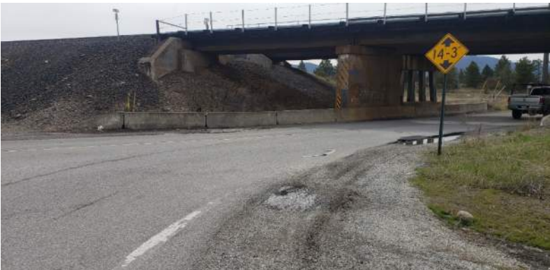
IMAGE 20: Starr Rd southbound looking at rail bridge, striping worn, shoulder ponding
