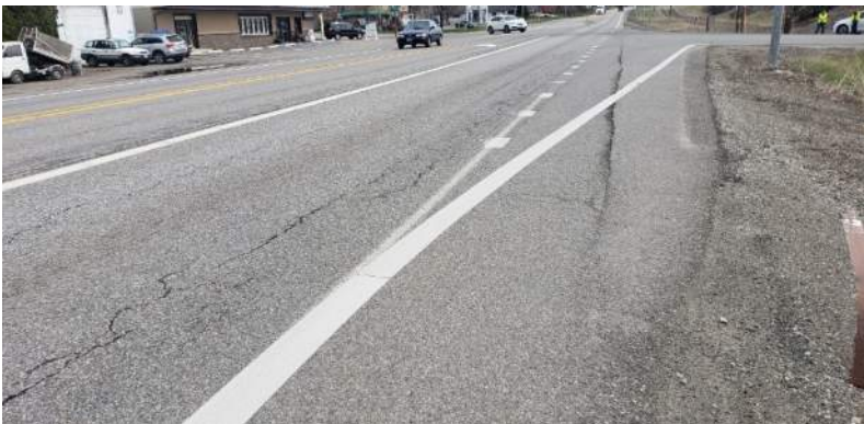
IMAGE 18: Trent Ave eastbound at Starr Rd, wheel path pavement cracks, short right turn taper
