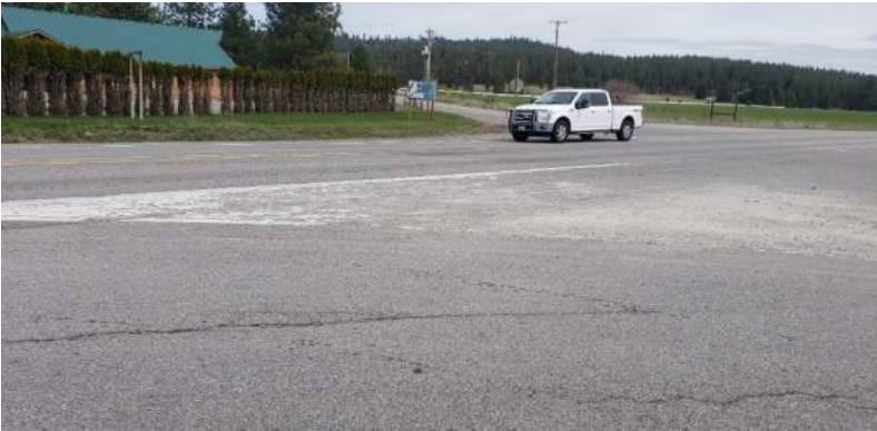
IMAGE 31: Trent Ave and Idaho Rd painted island hidden by gravel
